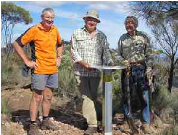
From left : Kevin, Modris, and Rob installing the new Topogram and platform for it on the Summit Viewpoint.
